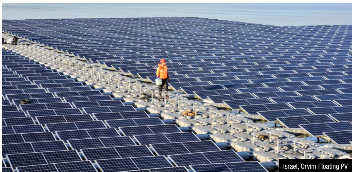
Israel, Revivim 2, PV + Storage
