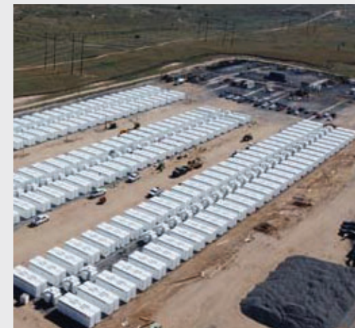
Atrisco BESS 1,200 MWh New Mexico
